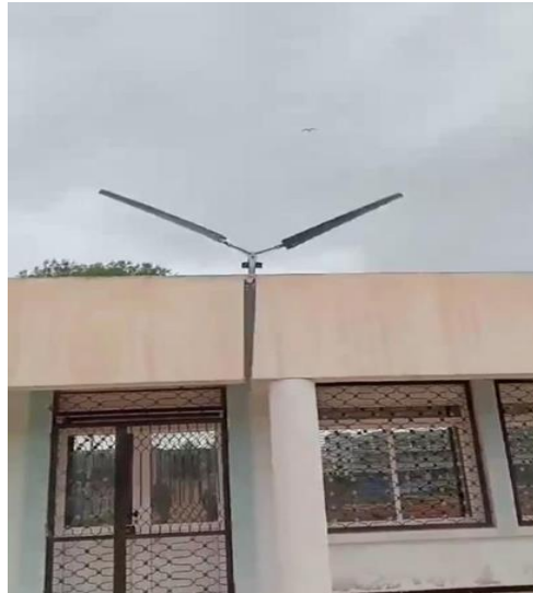
Fig.6. Prototype installation on the rooftop of the laboratory building for testing under natural wind conditions.
